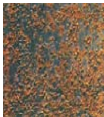
Steel surface with tinder starting to flake and first stages of rust infiltration
